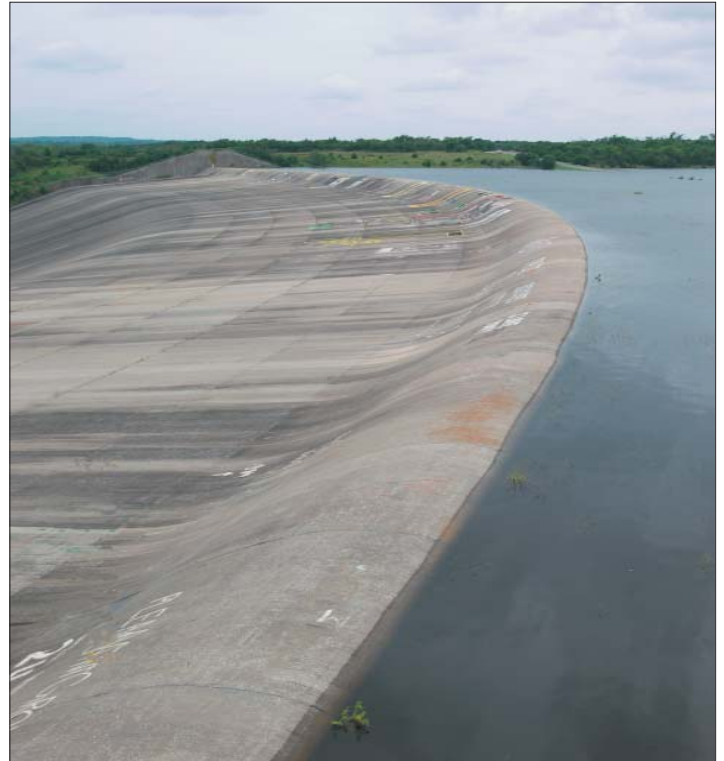
Lake Texoma's uncontrolled spillway is seldom used, but in July 2007, the lake reached the 640.0 elevation crest of the uncontrolled spillway. Shown above, the water level is just shy of flowing over. Sightseers came to witness the event which has only happened twice since the dam was completed in 1944.
