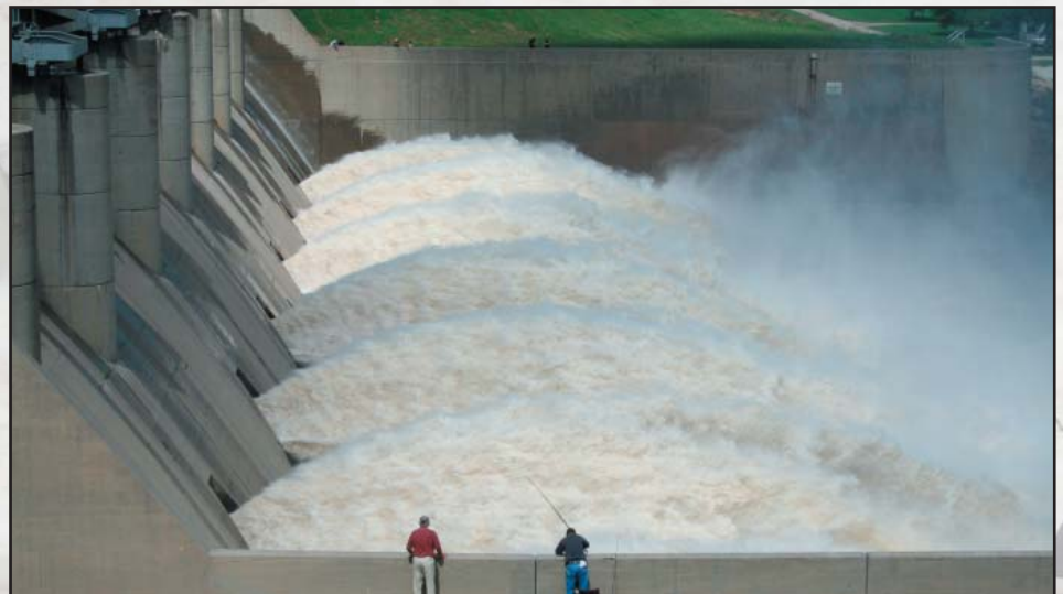
Fall River Lake, Kansas, (below) makes a spectacular scene as excess water is released through the spillway.
