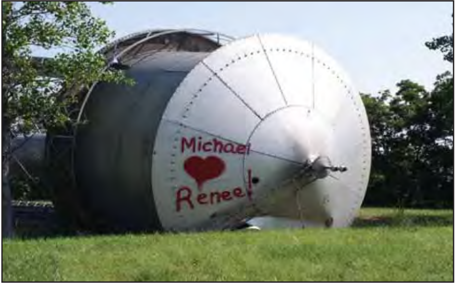
Everything is a canvas when you're young and in love. This is a shot of the water tower at Fall River after the demolition.
